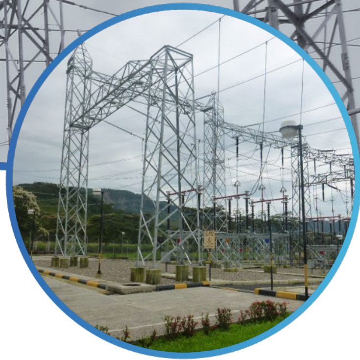
Detailed civil and electromechanic engineering and electrical studies: San Fernando and La Reforma substations 230 kV (Colombia) - Client: JE JAIMES INGENIEROS S.A.
