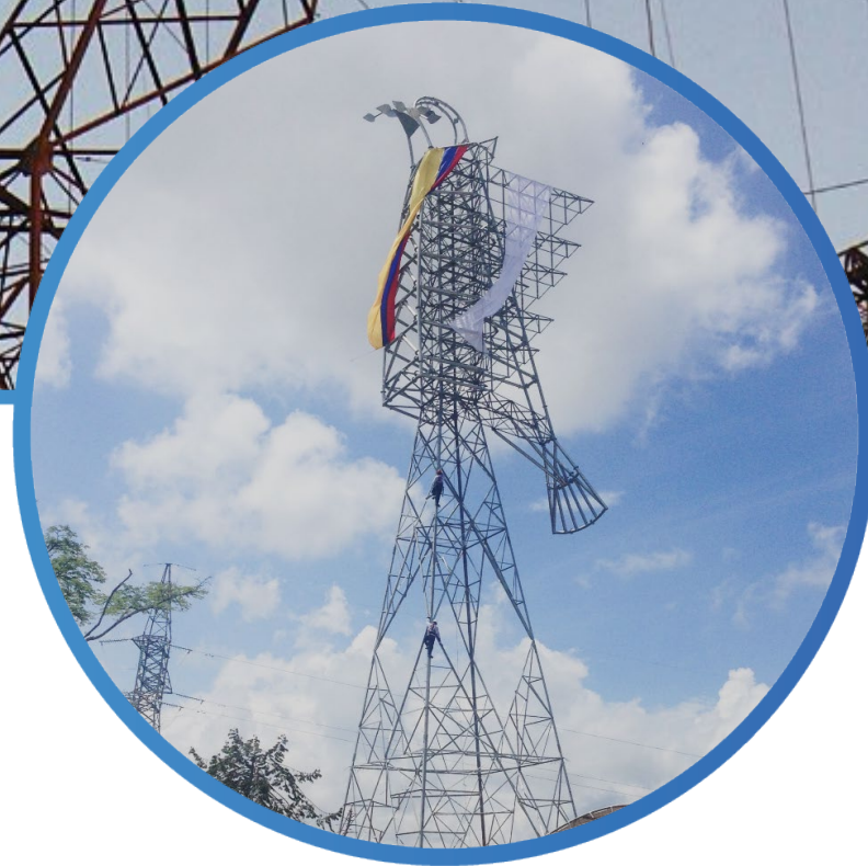
Detailed civil and electromechanic engineering and electrical studies: Tuluní connection Betania - Mirolindo transmission line 230 kV (Colombia) - Client: TUPROJECT S.A.S. ESP
